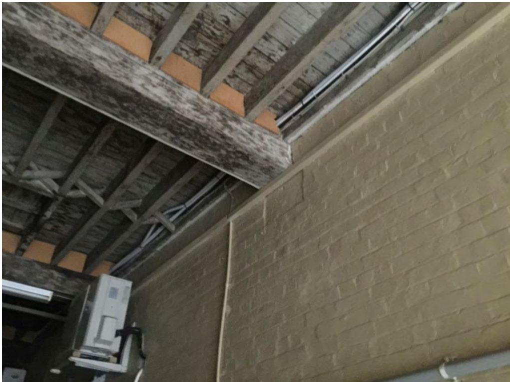
Figure 72 – Timber beam borne on stone block in wall of Cartway (Y01) NBRS+Partners, April 2015.
