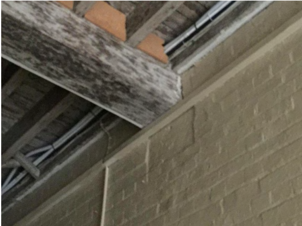
Figure 73 – Timber beam borne on stone block in wall of Cartway (Y01) NBRS+Partners, April 2015.
