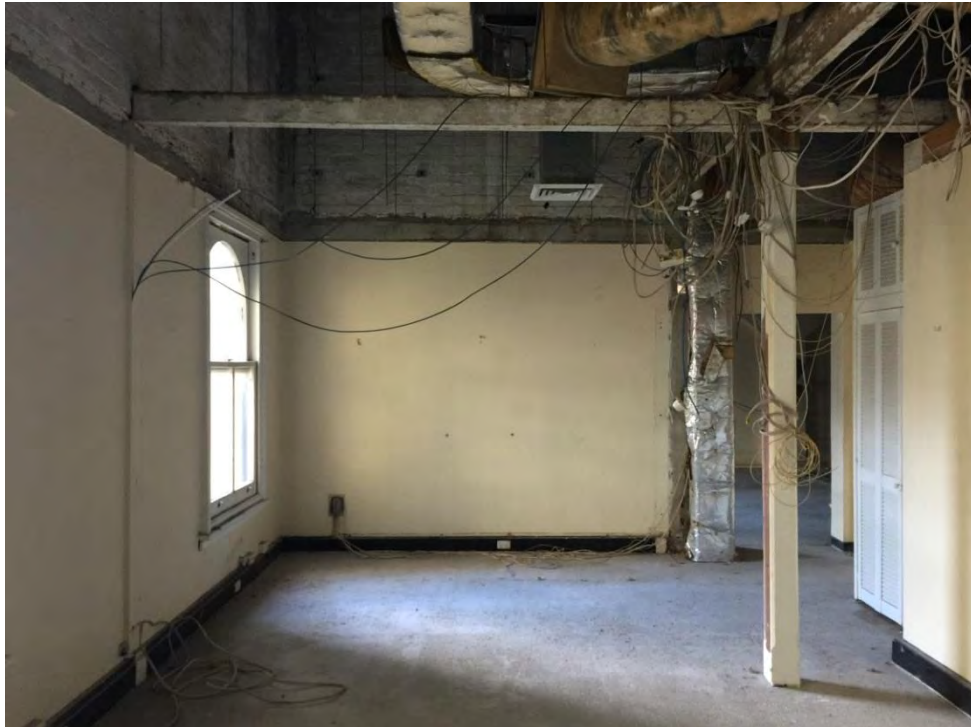
Figure 93 – Western section of space S02 showing timber post, beam and truss structure. NBRSPartners, April 2015.
