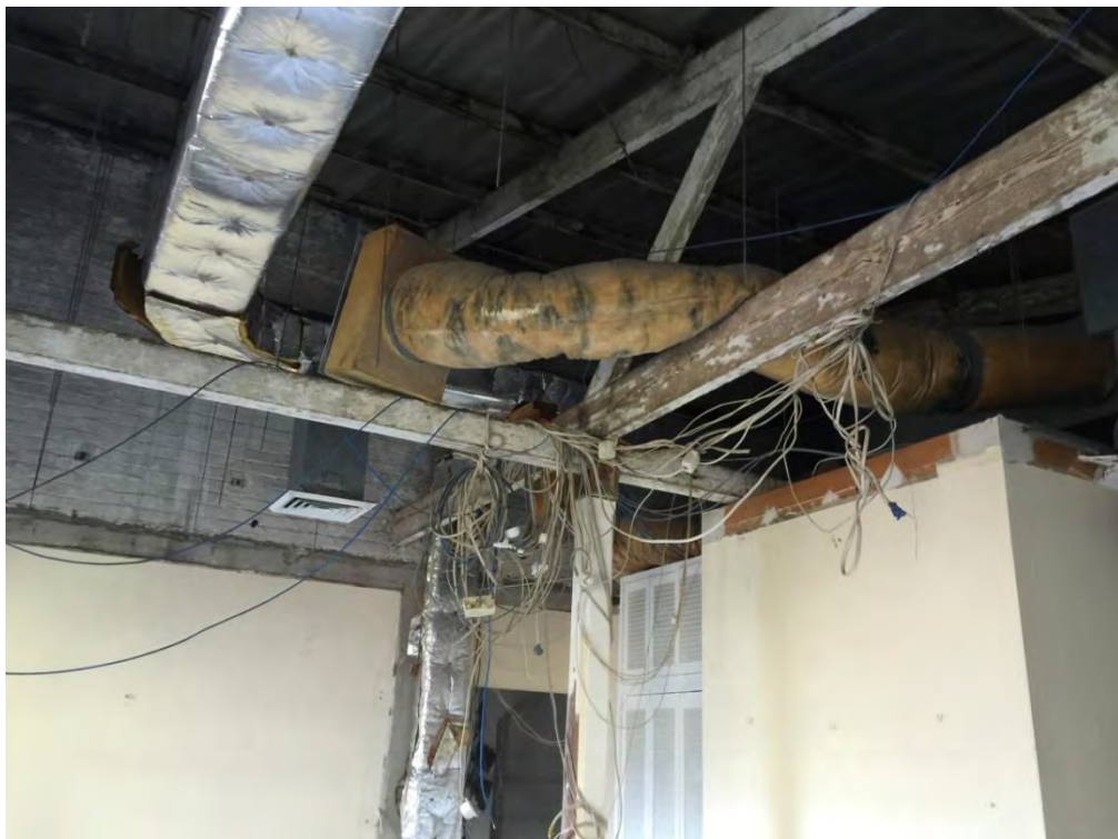
Figure 94 – Western section of space S02 showing timber post, beam and truss structure. Recent studwork walls to stair and service core at right. NBRSPartners, April 2015.
