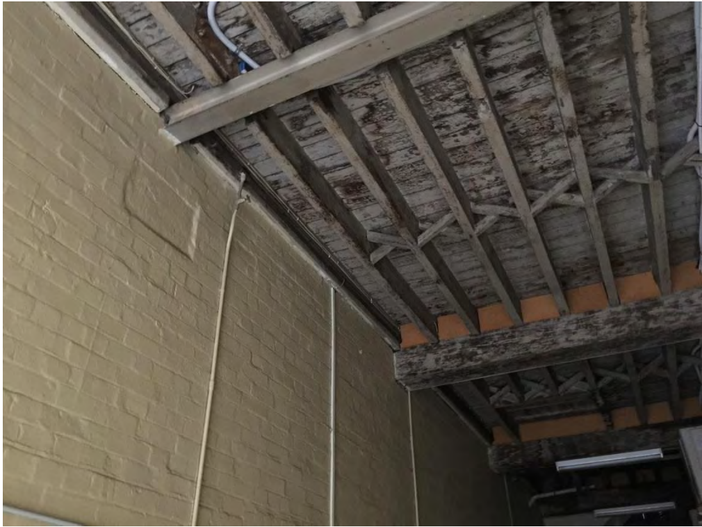
Figure 71 – Steel beam in place of timber beam borne in wall of Cartway (Y01) NBRS+Partners, April 2015.
